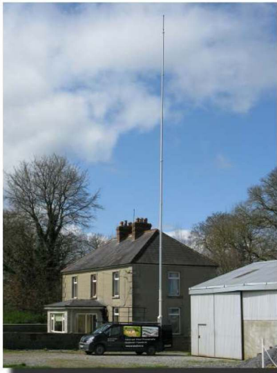
Above, note the height of the mast in relation to the two storey house
